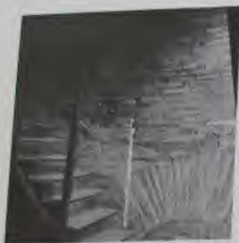
Fig. 300. S. Sustina. South wall of nave, (restored), showing masonry and "restoration" work in the area of window.
